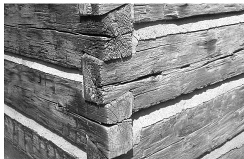
Figure 4.—Close up of southeast corner of the Grayson house showing half-dovetail notching.
