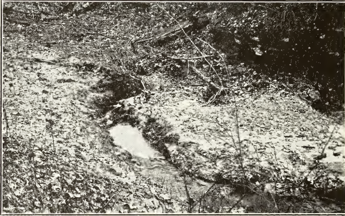
Fig. 5—The sink inlet for Myers Branch. Note accumulation of trash and debris surrounding inlet.
