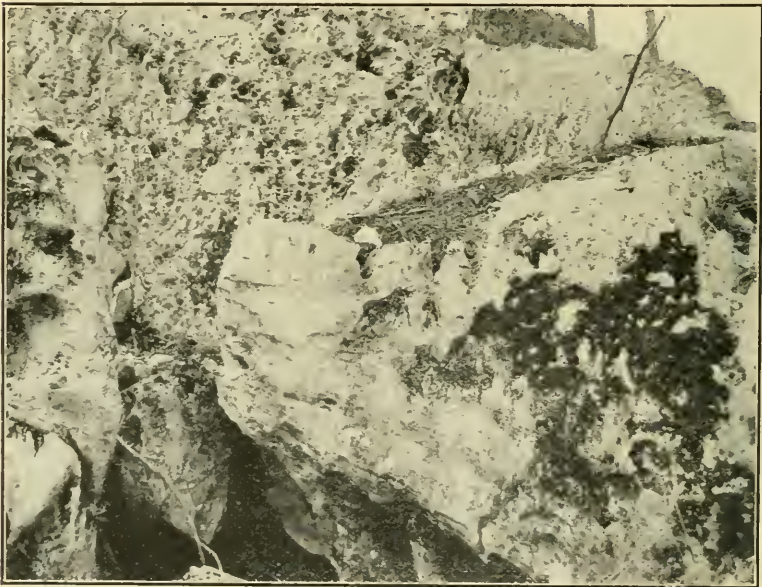
No. 6. Detail of a portion of No. 5, showing honeycombing.
